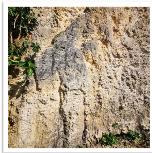
Figure 5. Crack or discontinuities condition on the rock mass in the Melasti Beach area
