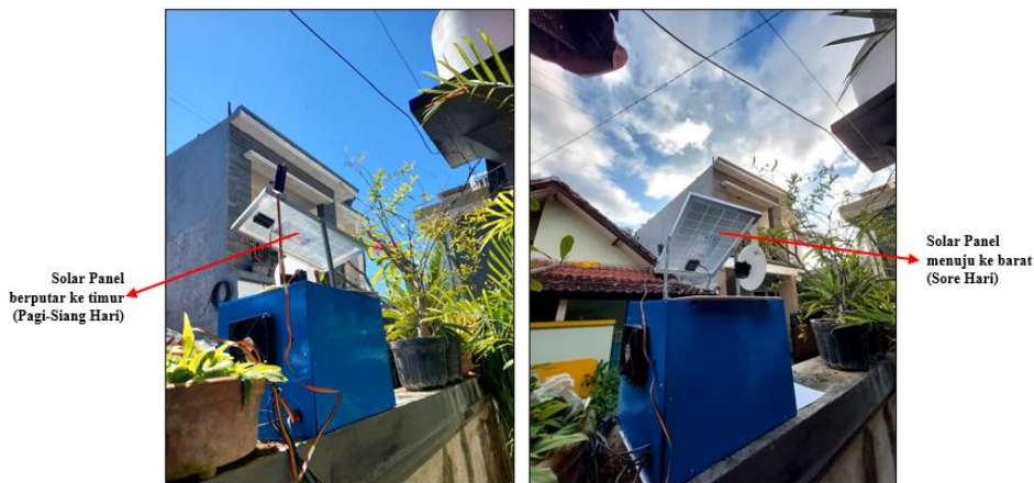
Figure 8. Testing Monitoring and Solar Tracking System
