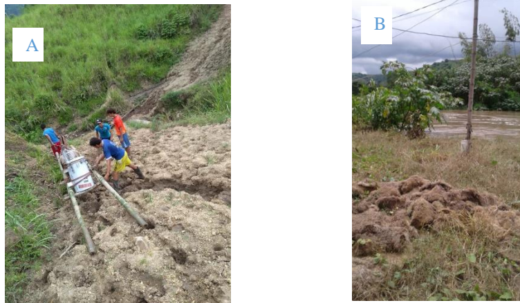
Figure 2. Images of the adverse conditions of the Guillen creek
